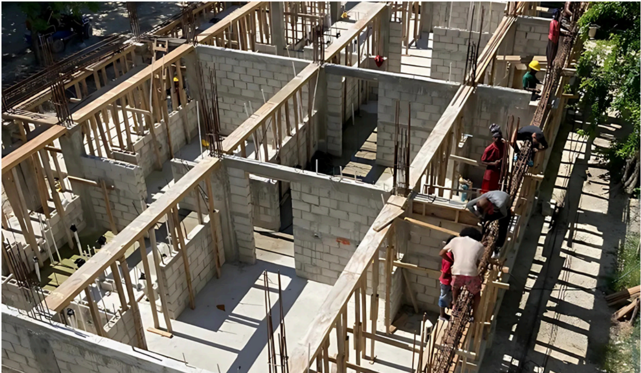
Construction photos of the Galleon building at Grand Baymen Gardens in Belize as of December 2024.
