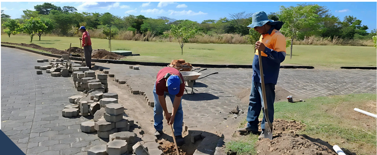
Construction photos of the CLARO fiber installation at Gran Pacifica in Nicaragua.
