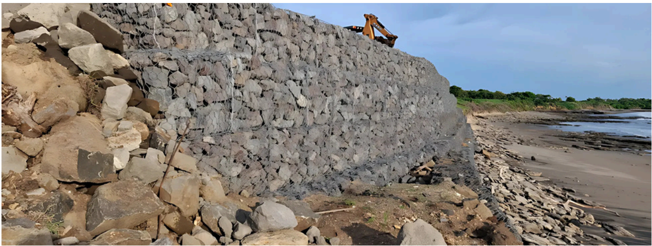
Construction photo of the gabion installation along the Gran Pacifica (Nicaragua) shoreline to mitigate erosion.
