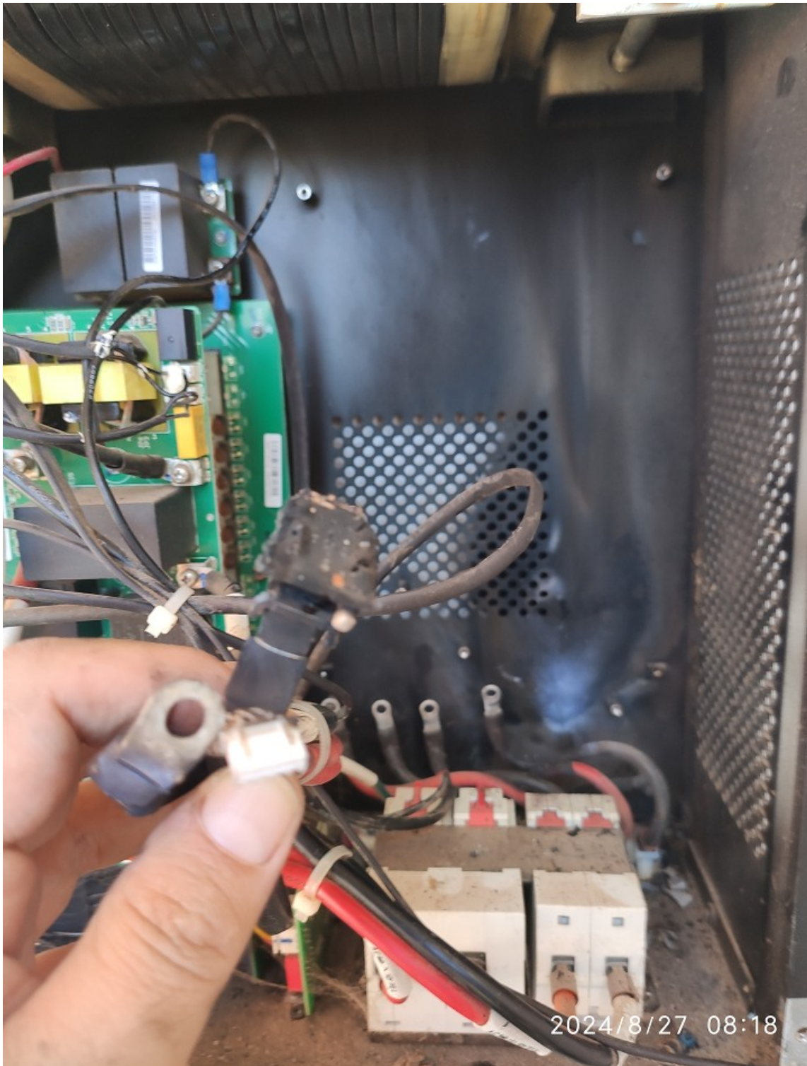
IMAGE 2 OF INVERTER / FIRE
